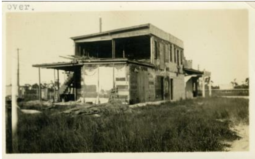
over. Harry Hull Home, Jupiter Florida - Sept 3, 1933 — Hurricane did this — Blew the ends out of 2 bedrooms as shown, part of furniture in field; there was a 2-story porch on front which is gone; blew out all doors and windows, there was another apartment on the end from Martha's and garage underneath.
